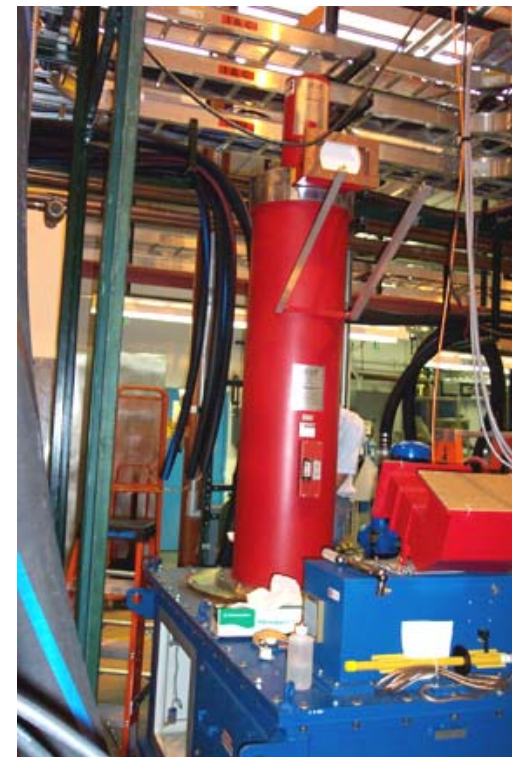
Tube installed in transmitter at Los Alamos
