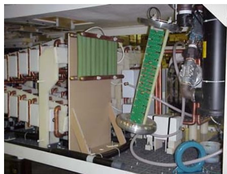
Oil Pump & Voltage Divider
