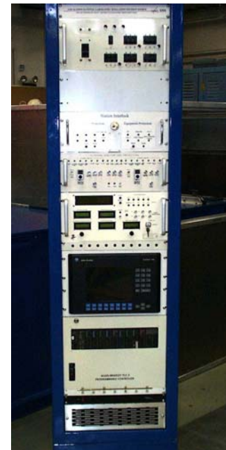
EQUIPMENT CONTROL RACK
