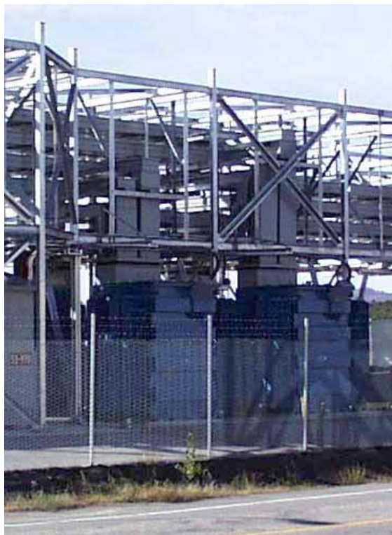
Typical H.V. Transformer
