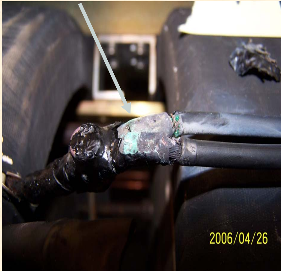
Melted Electrical Tape and Corroded Magnet Connections
