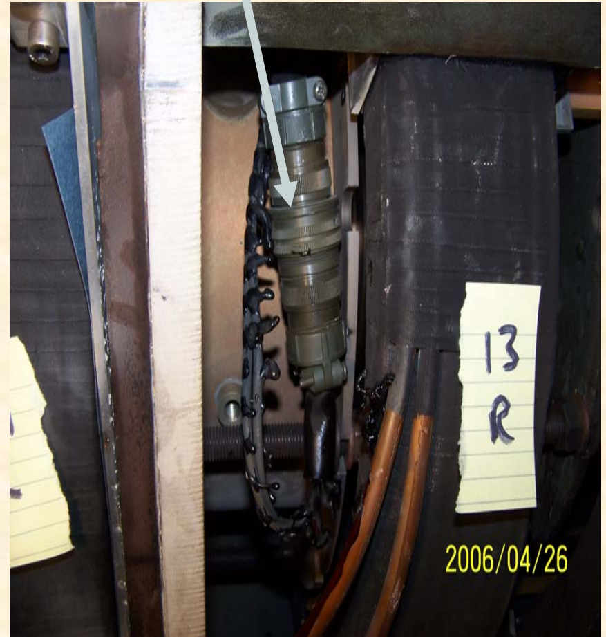
Short May Have Started By Water Leaking into This Connector
