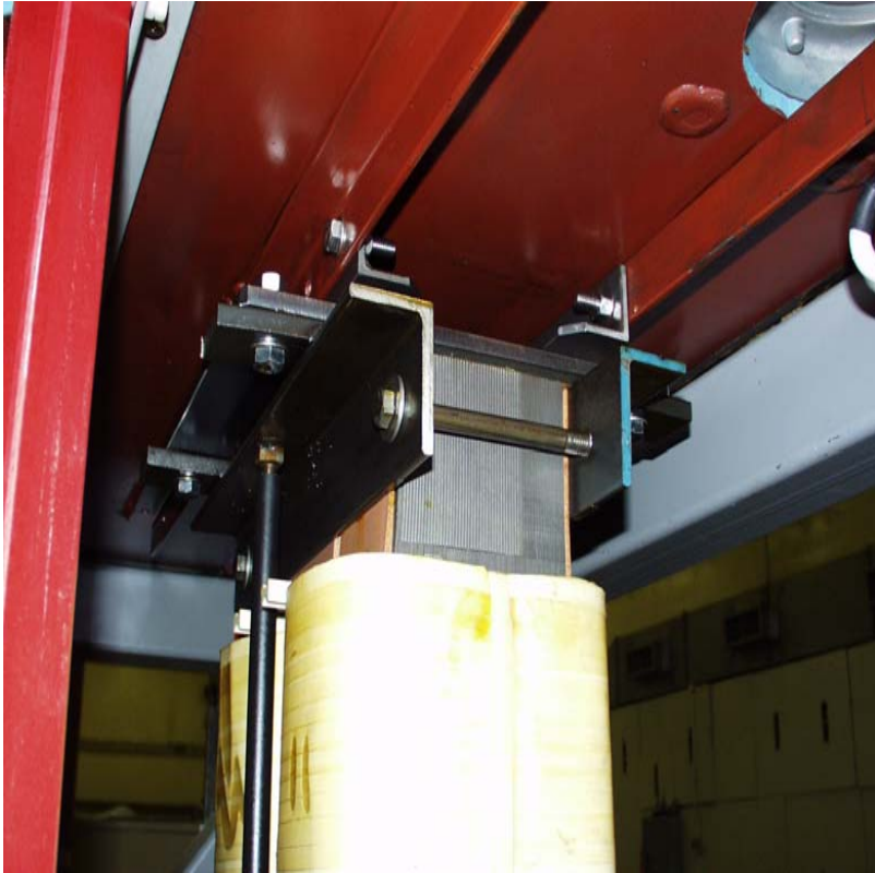
Interphase transformer mounts were checked for tightness
