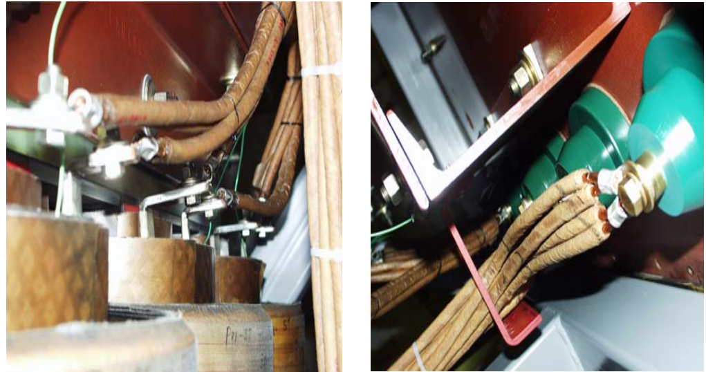
400v primary connections were checked for tightness and evidence of overheating
