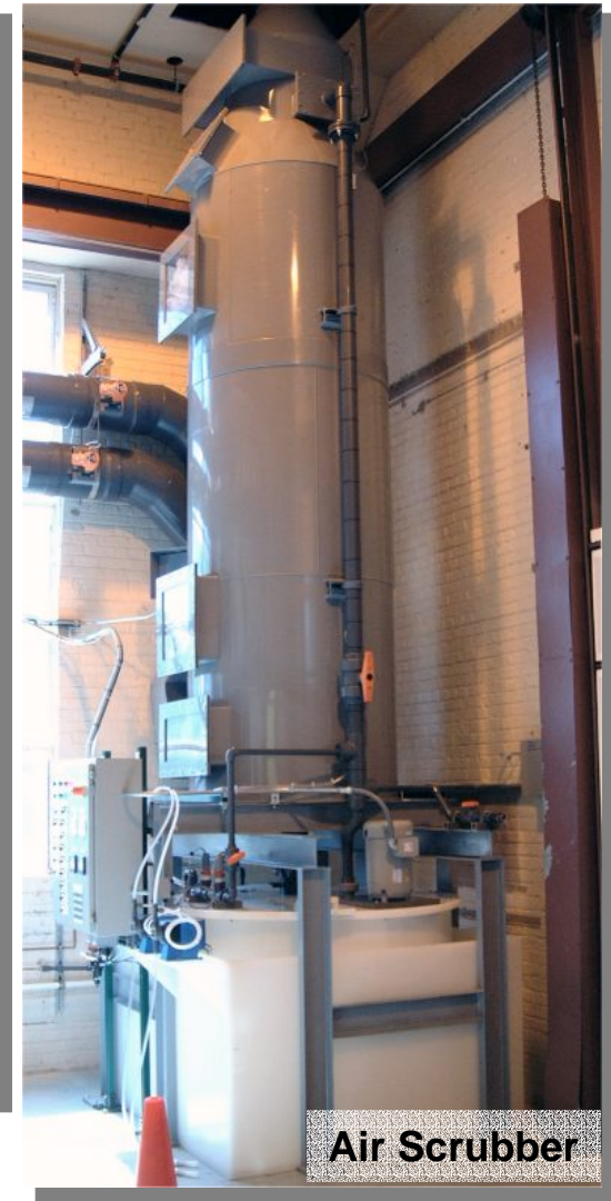
Chemical Processing Rooms
