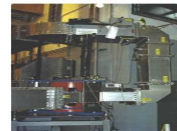
Acceptance Test of Waveguide Shutter at 1 MW RF Power Using RF Circulator.
