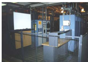
RF1 Station Powering RF Test Stand.
