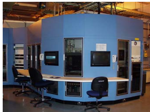
RF test stand operator console.
