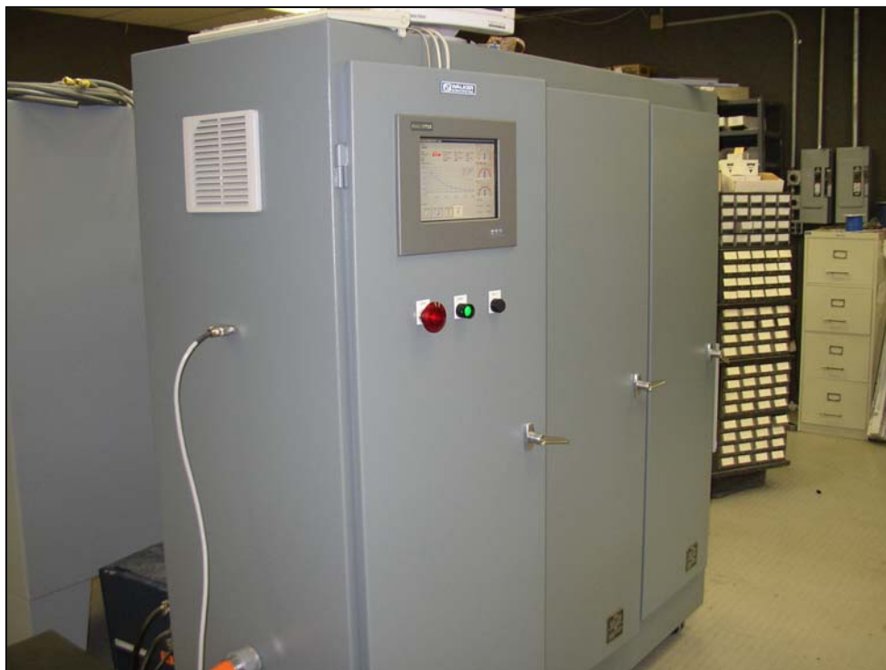
Power supply and control system
