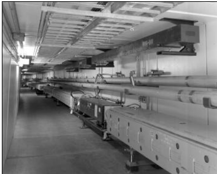
Figure 2. Recycler gradient models hang from the ceiling above Main Injector magnets
