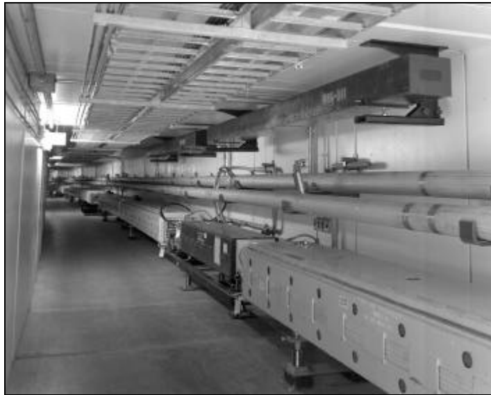
Figure 2. Main Injector magnets Recycler gradient models hang on the ceiling
