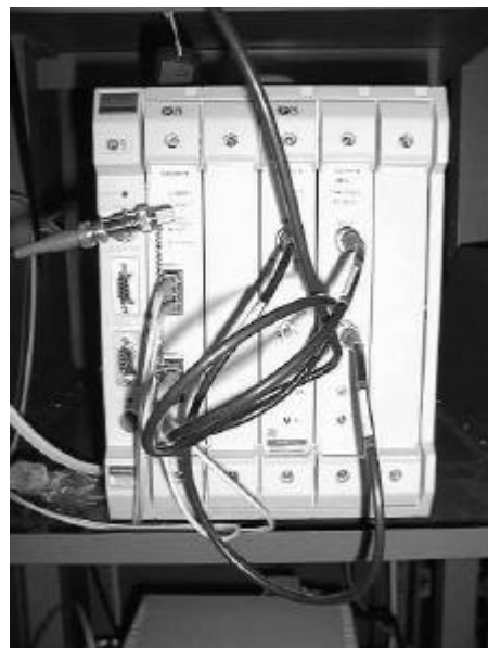
Figure 5. WE7000 station. From left, station power supply and RC232C interface, optical fiber network in/out and four modules.
